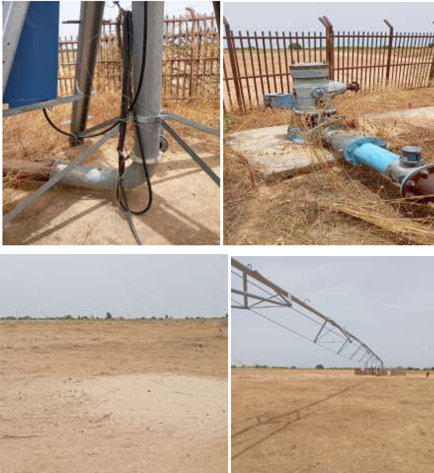
Plate1.0. The Project site being used for grazing and with collapsed Telecommunication mat Infrastructures inside
