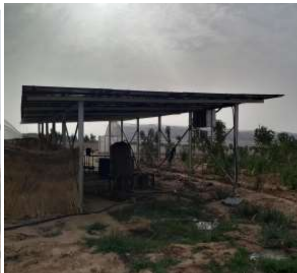
Solar farm (10kW)
