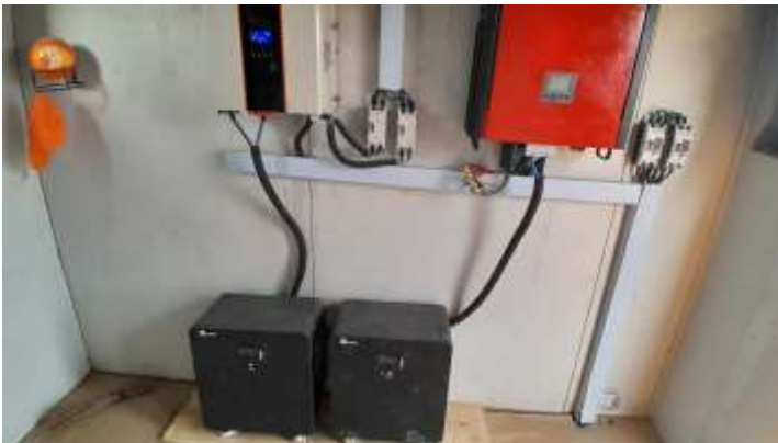
10kW each battery inverter (2pcs)
