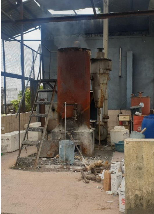
Plate 5: Waste Incinerator at LUTH
