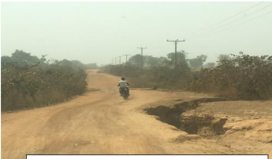
Figure 3: Section of R2-3 showing one of the river crossing Observed cutting across sections of the Road
