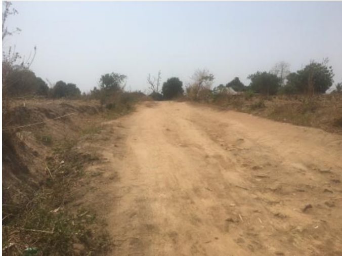
Figure 4: Wideness condition of some of the roads, indicating No Potential Involuntary Resettlement
