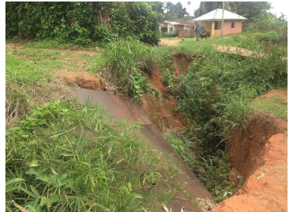
Plate 8: A failed crossing platform at a section of the erosion
