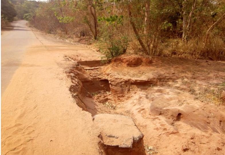
Plate 4.14: Ewu Monastery Road Devastated by Growing Gully Erosion
