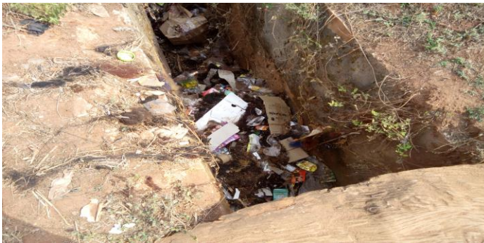
Plate 4.11: Waste Deposition in Drainage Channels
