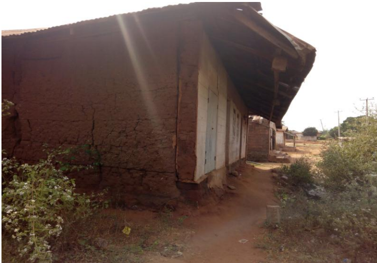
Plate 4.24: Structurally Affected House Close to the Gully Head in Ewu Town
