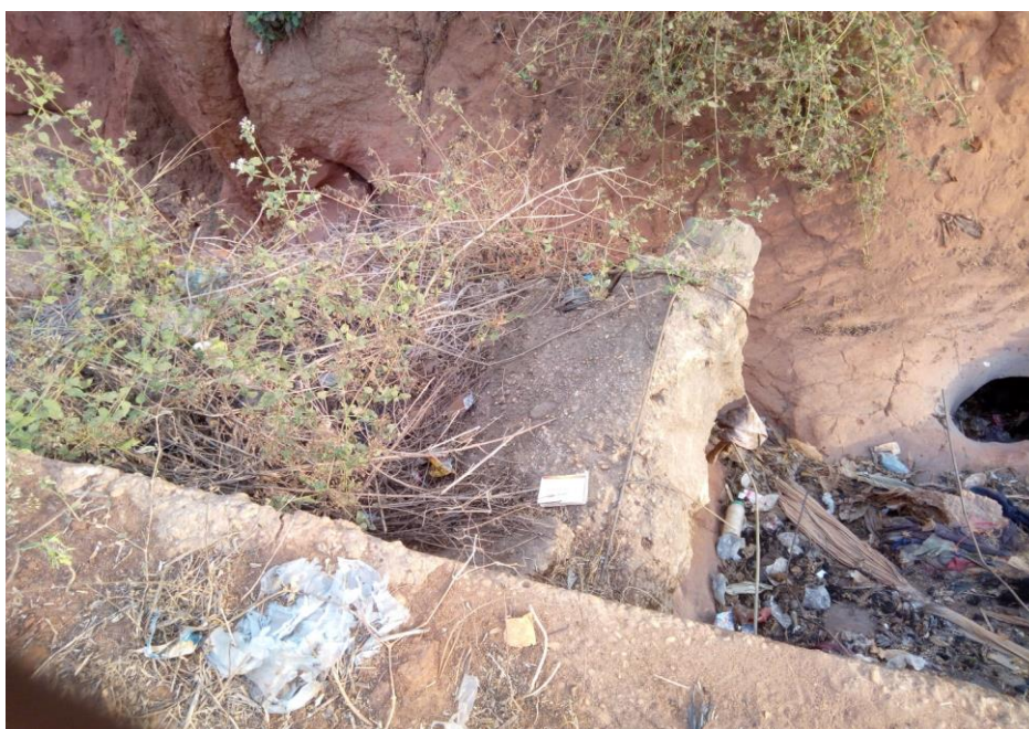
Plate 4.5: Waste Deposited Inside the Gully Site
