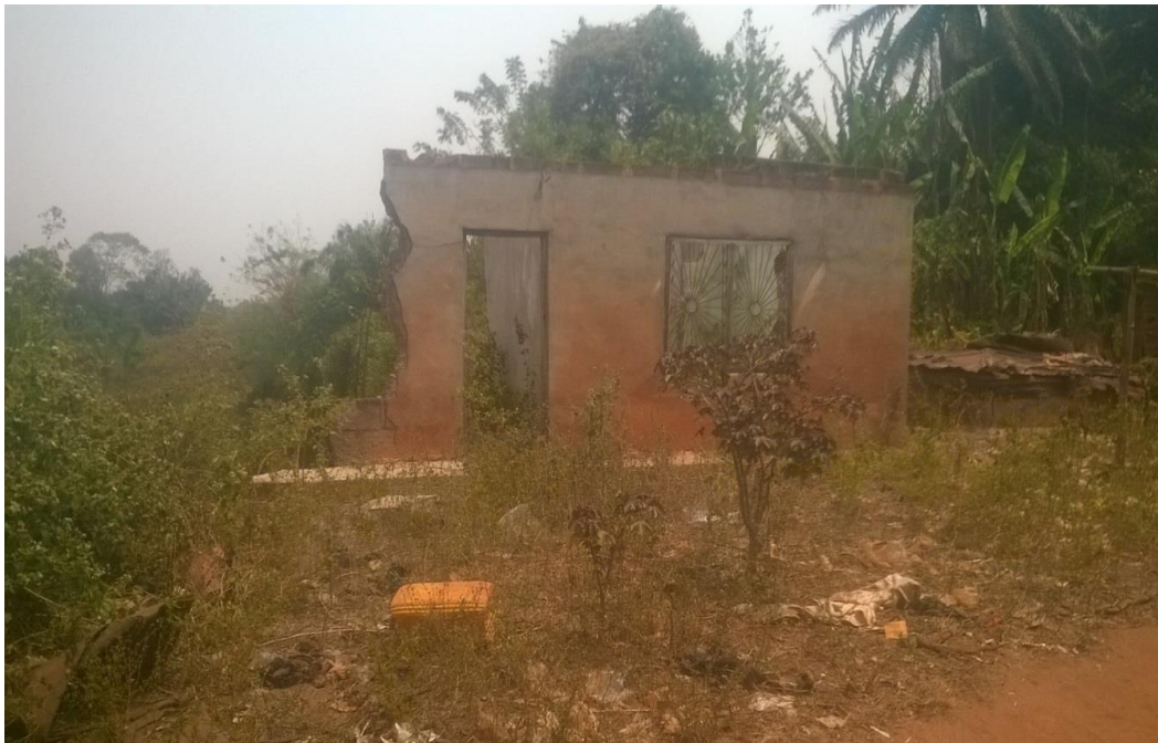
Plate 3.4: A collapsed building at Ibore gully head.
