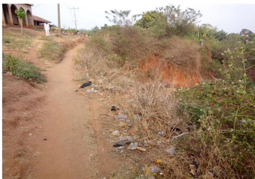
Plate 4.6: Gully Encroaching into Road in Ibore Community
