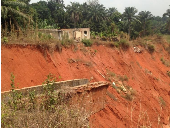
Plate 3 Collapsed Concrete Canal
