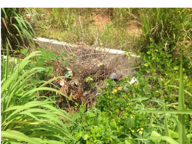
Figure 6 Broken drainage on Ngwo-9th Mile Road
