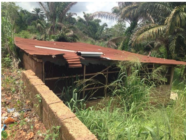
Figure 10 Part of a poultry house damaged by the gully
