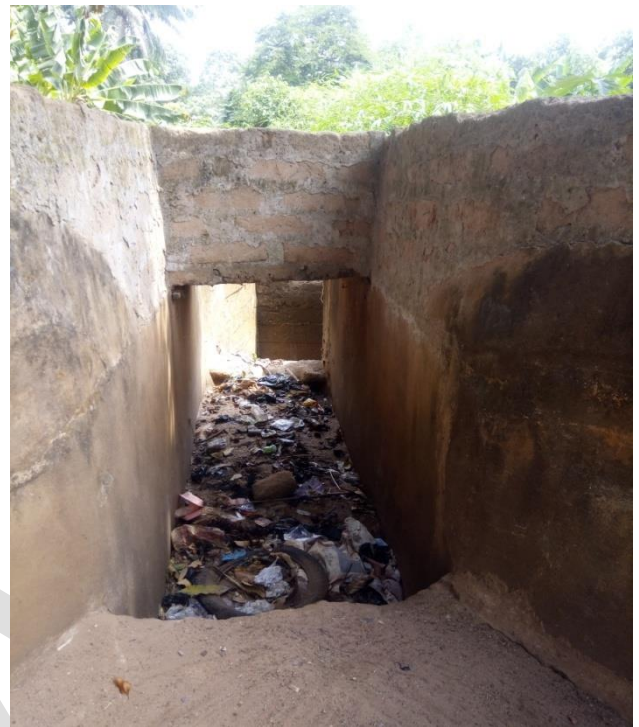
Plate 3.3:: Failed Drainage Channel at Ire Obosi
