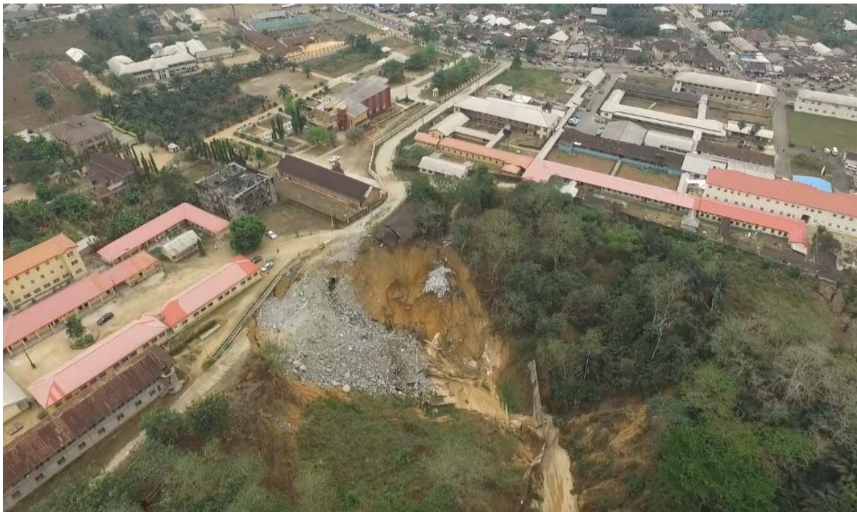
Arial view of the St. Luke's Hospital gully erosion site
