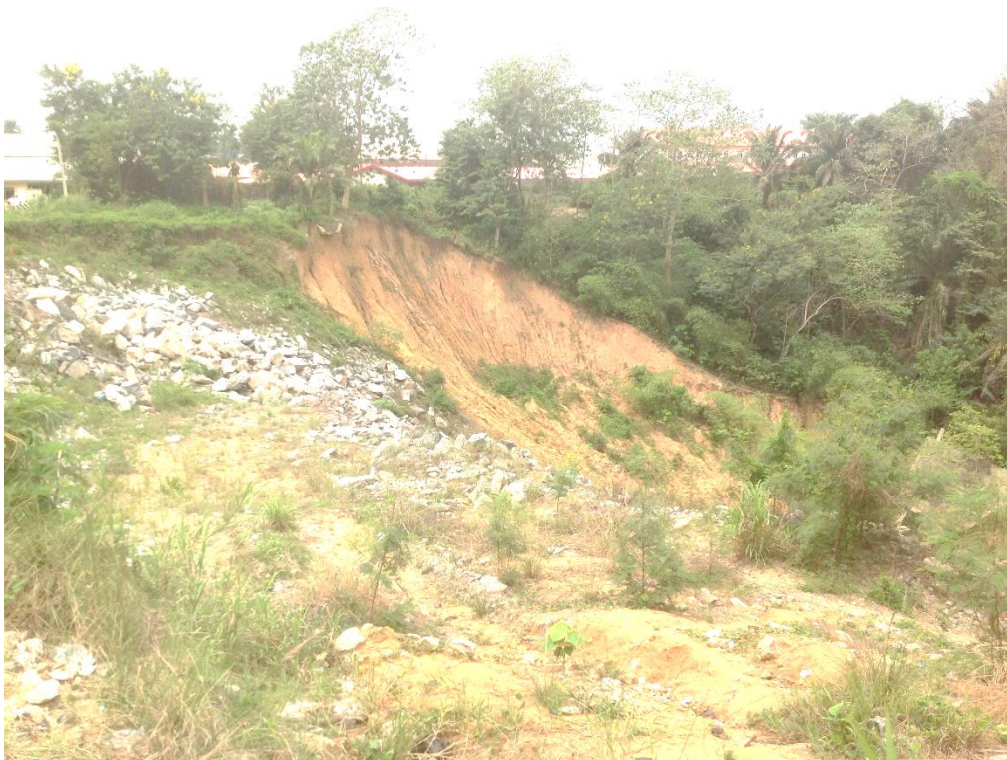
Plate 3.2: Active gully erosion threatening economic trees and buildings
