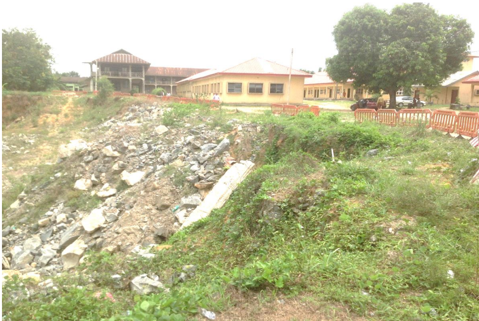
Plate 3.5: Several buildings are at risk of collapsing into gully channel
