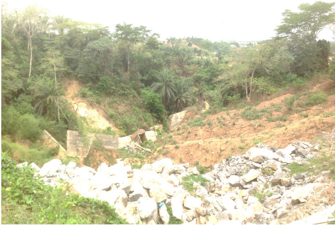
Plate 3.3: Previous Remedial Civil Works at St. Luke's Hospital Anua Gully Erosion Site Collapsing into the gully.
