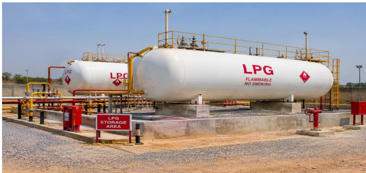
Figure 3.2: Storage System of LPG
