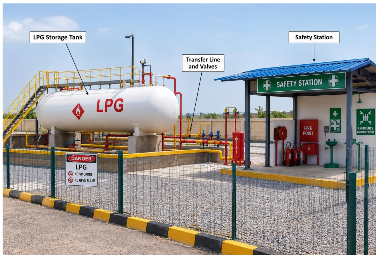
Figure 3.4: LPG Storage Facility with Safety Station
