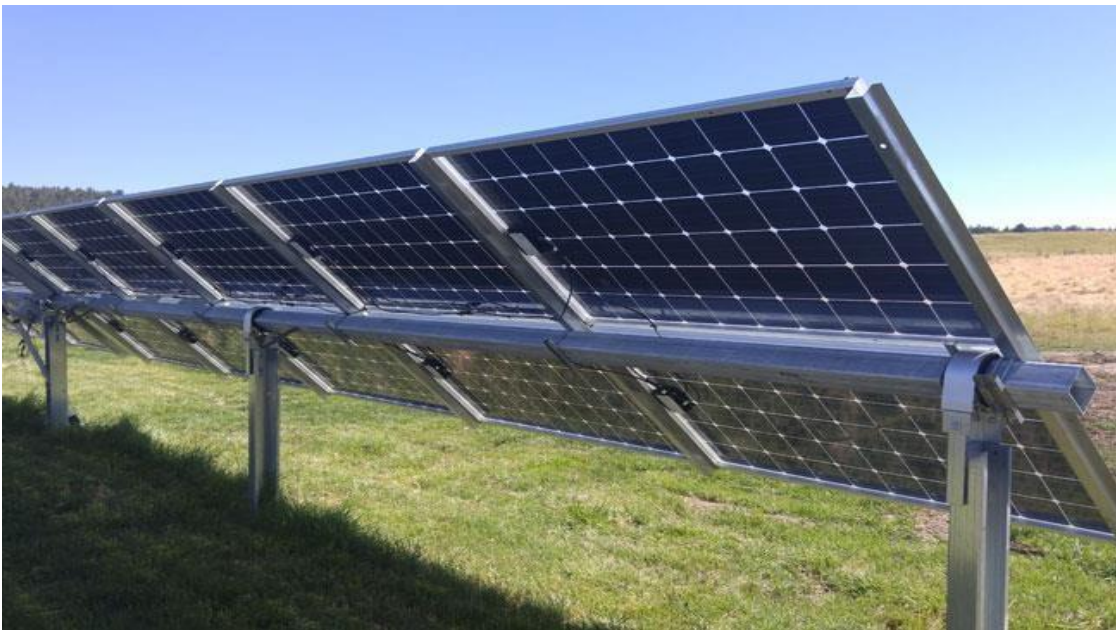
Plate 2.4: Bifacial Solar panels
