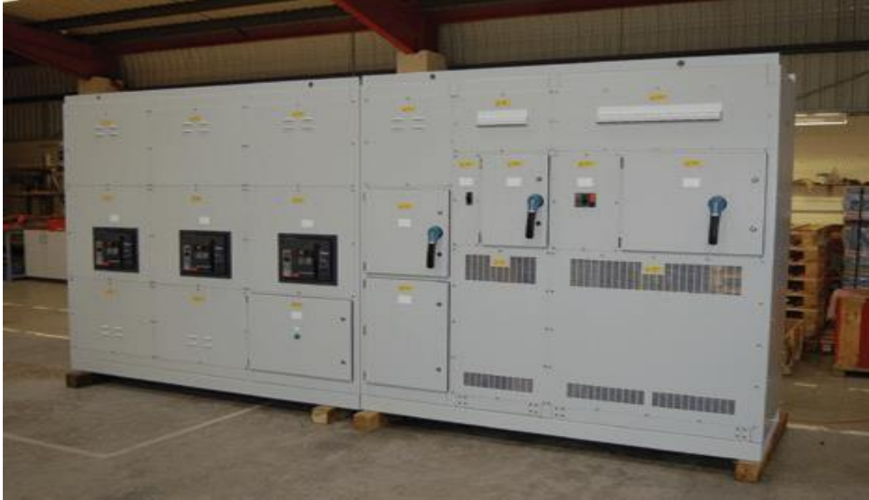
Plate 3.2: A typical low-voltage switchgear cabinet.
