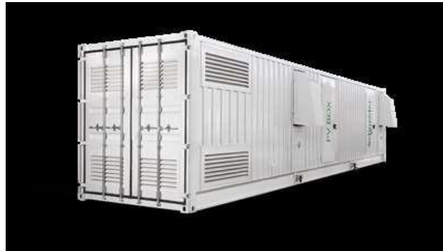
Figure 3. 8: Example of a power station (Source: REA EEP 3 FEED)
