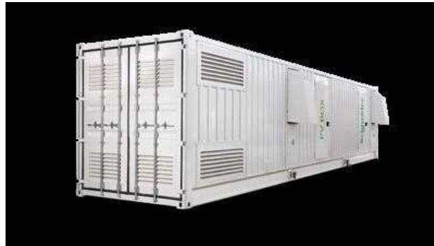
Figure 7: Example of a Power Station
