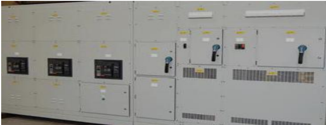
Plate 3.6: Showing a typical switch gear cabinet
