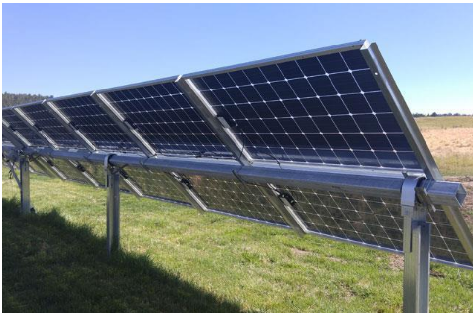
Figure 2.5: Bifacial Solar panels
