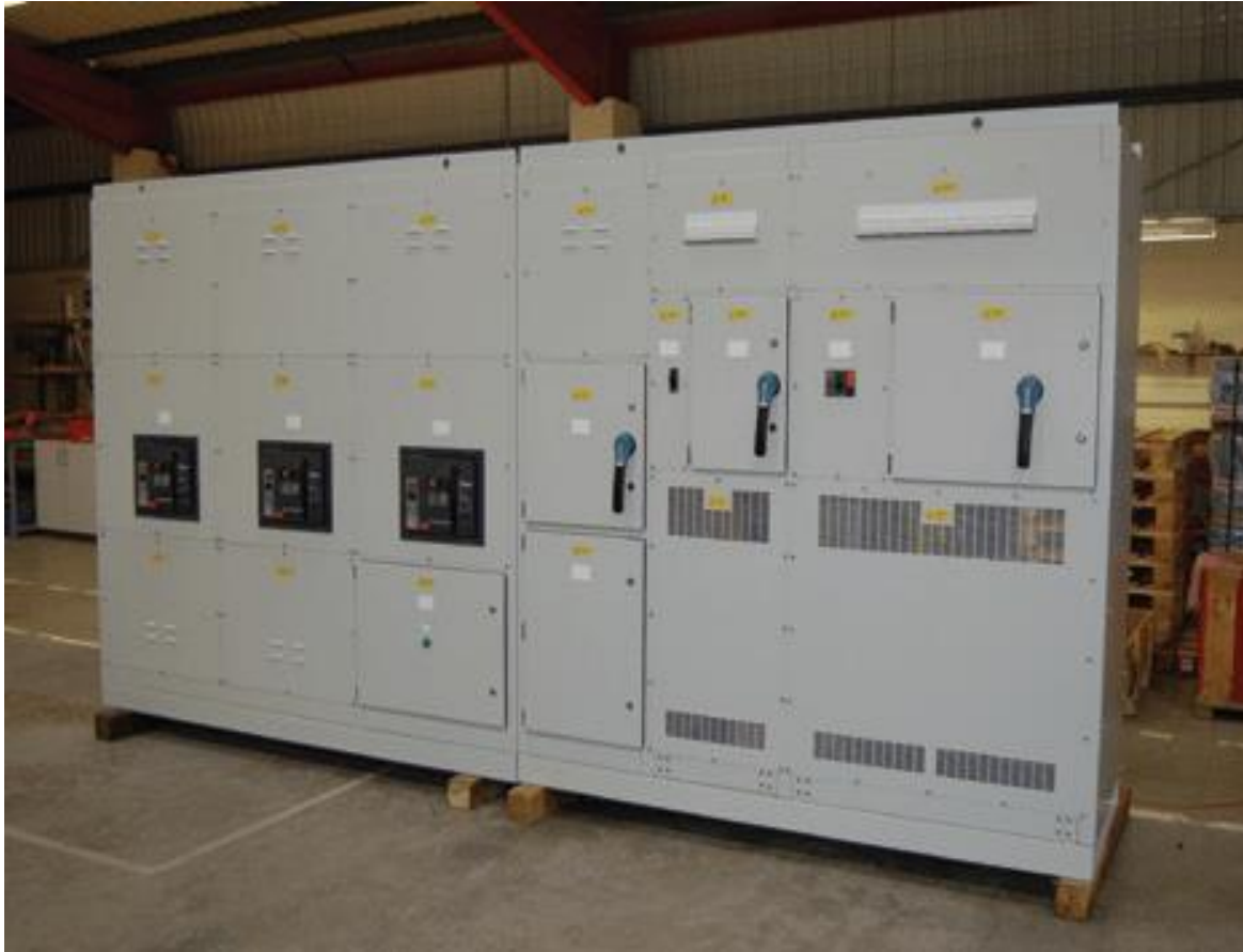
Plate 3.4 A typical low voltage switchgear cabinet
