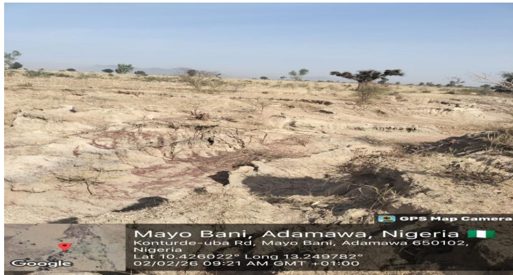
Figure 19: Evidence of Surface Erosion within the Proposed Project Site, FUAMB, Mubi
