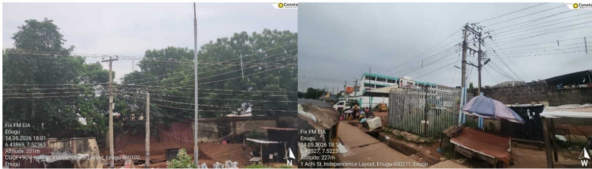
Plate 4.14: Power Transmission Lines and Transformer in the Study Area (Source: FIX FM 103.3 MHz Field Studies)
