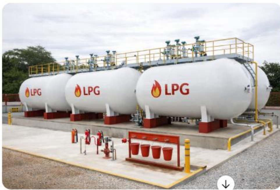
Figure 3.5: LPG Storage Facility with Safety Station
