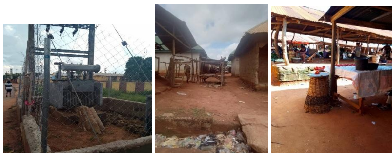
Plate 4.18: Electric Power Infrastructure in Ipuole Okuku village (left)
