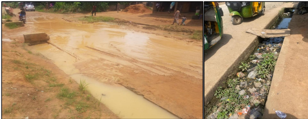
Figure 8: Waterlogged Drains in Obingwa LGA—(Left) Overtopped Drainage Channel, and (Right) Deposition of Municipal Wastes into Existing Drainage at Umuariama – Ahiaba Ubi – Nkwo Elechi Market Road, Obingwa LGA
