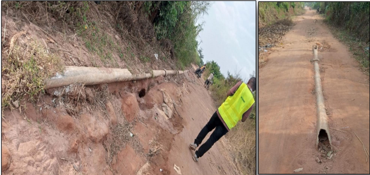
Figure 13: Buried Asbestos Pipes Exposed/Protruding Along the Nbawsi – Agburuike – Umuomaighiukwu Road (Upgrade, Lot 3)
