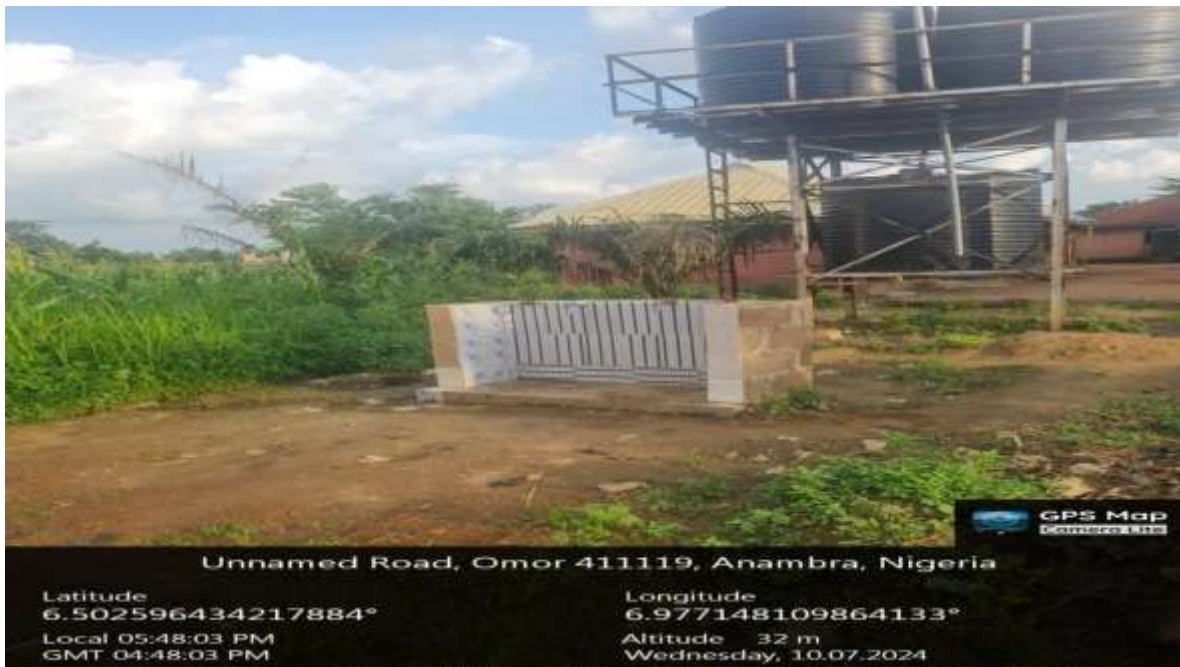
Plate 4.20: Community Borehole in Omor Town
