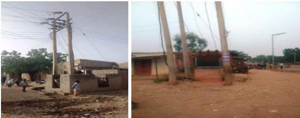
Plate 4. 36: Electricity transformer at Zangon Kaya Ungogo LGA (left) and electric poles and strung lines for electricity supply at Gwarabjawa, Danbatta LGA (right)
