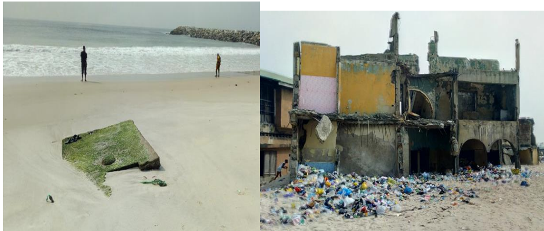
Plate 4.9: Submerged and damaged building at Alfa Beach, Eti Osa LGA
