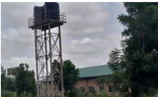
Overhead water tank
