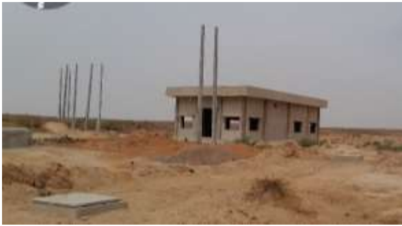
Electrical control room/sub-station
