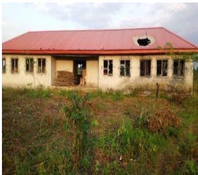
b. Non-functional health facility at Obodougwa
