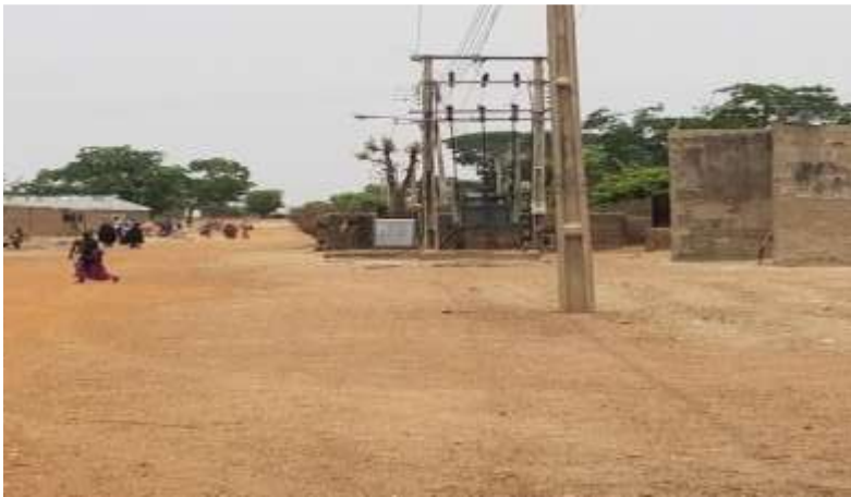
Plate 1.23: Transformer that supplies the communities with electricity, located at Kuhu
