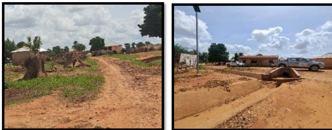
Plate 4. 5: Some Parts of 10Km Patishin-Danko-Masallaci Road without and with Drainages
