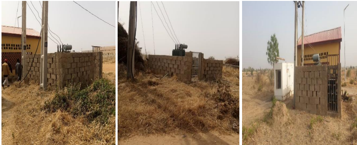
Plate 2. 3: Existing Transformers in FUDMA (Source: Field Survey for the proposed EEP 3, July 2022)
