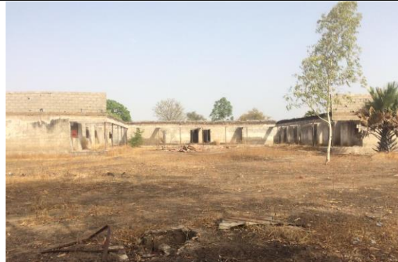
Burnt down buildings in the school due to insurgent attacks
