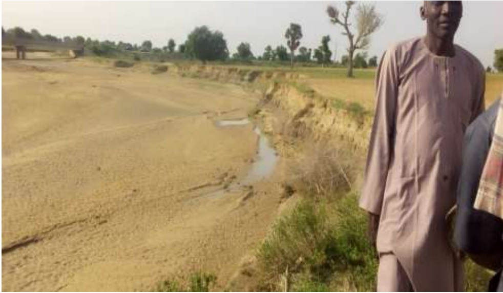
Plate 3.2: Riverbank Erosion and damage to critical infrastructure in Challawa Gorge Dam Watershed Area (July 2021)
