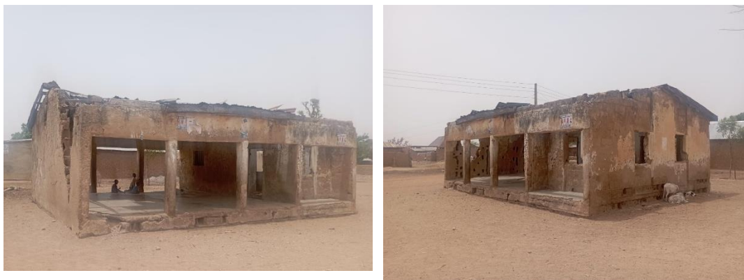
Plate 7.4: Dilapidated and Abandoned PHC in Tsara Chikin Gari community
