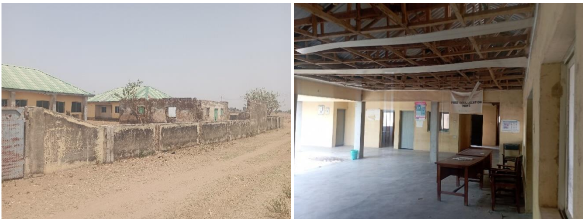
Plate 11.1: Dilapidated Health care center in Tsara Chikin Gari Community
