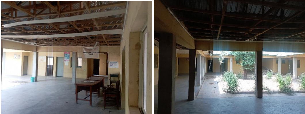
Plate 7.3: Dilapidated PHC in Tsara Chikin Gari community
