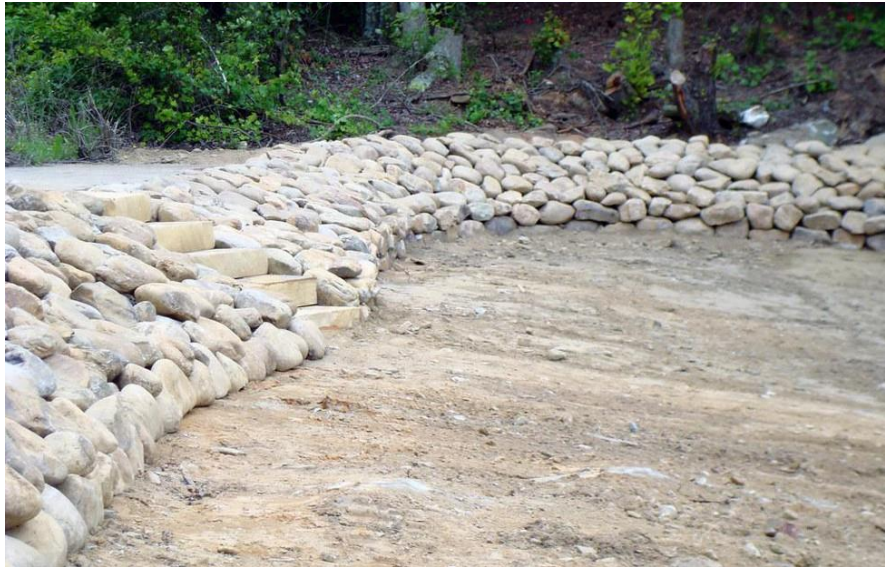
Plate 3.3: River Rock Riprap for Stream Bank Erosion control
